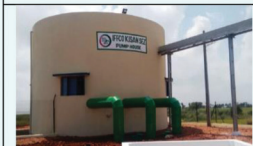
Pump House at Kanigiri Reservoir
